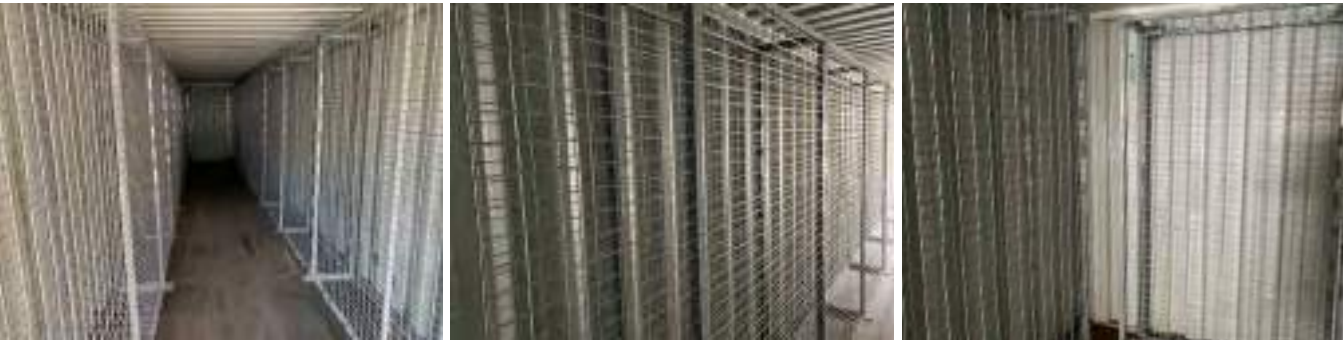
Mesh Racking in a 40ft Container.
